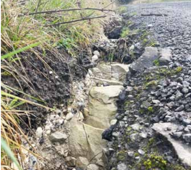
Roundway rain damage
